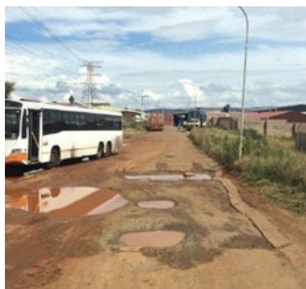
Potholes in Nancefield
